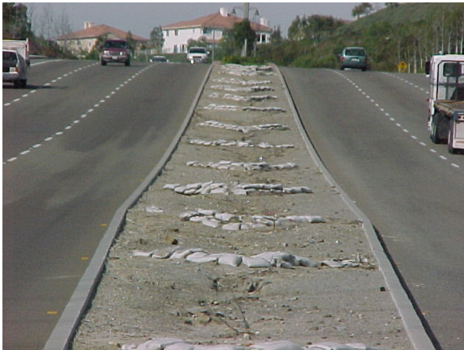
Sandbags were placed on Oso Parkway several years ago and continue to control erosion in the median
