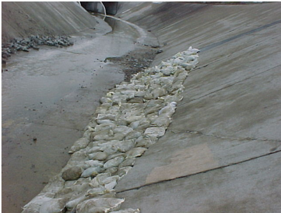
Damaged lining on E05 U/S Orangethorpe L/S
