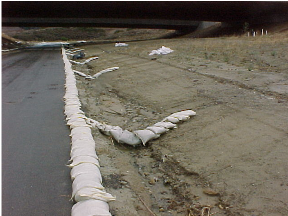
Chevrons and a row of sandbags placed along an A/C roadway for erosion control
