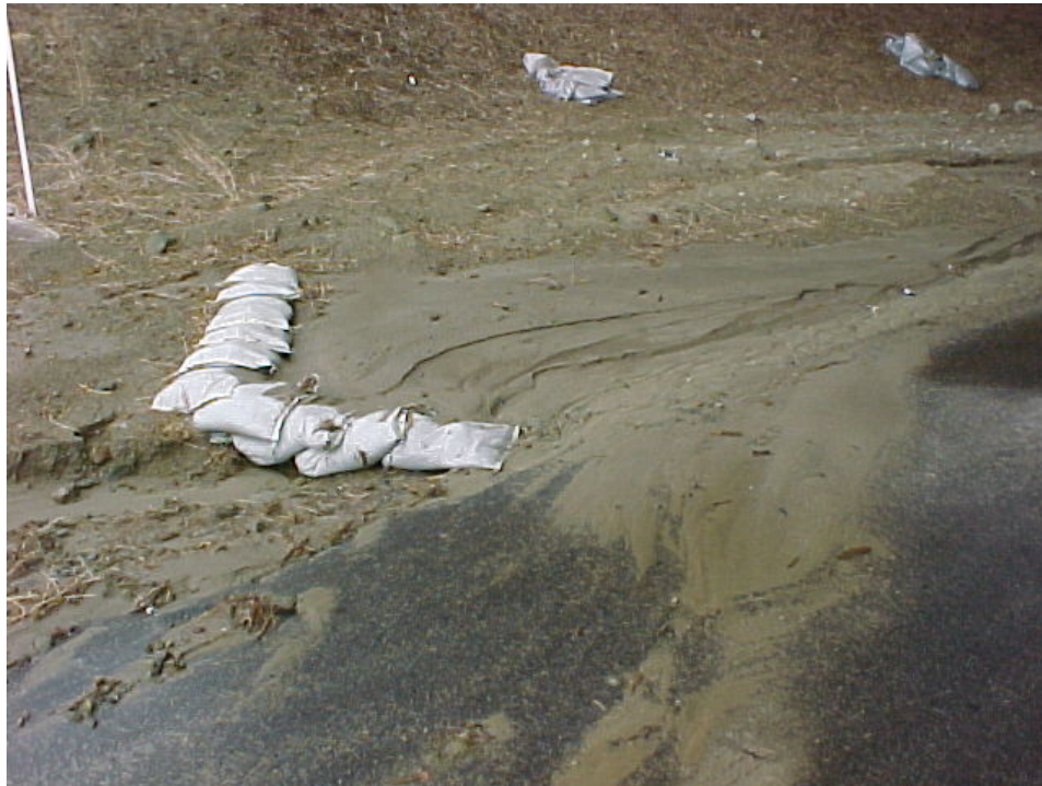
Erosion control using sandbags placed as chevrons. Note the silt building up behind sandbags spilling into roadway
