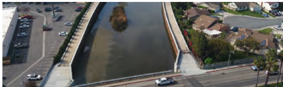
East Garden Grove-Wintersburg Channel and Ocean View Channel system is one of the underlying channel systems that does not currently have the capacity to contain the 100-year flood as the channel banks and levees have over-topped at several locations.
